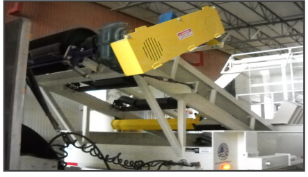
42" Under Crusher Conveyor
